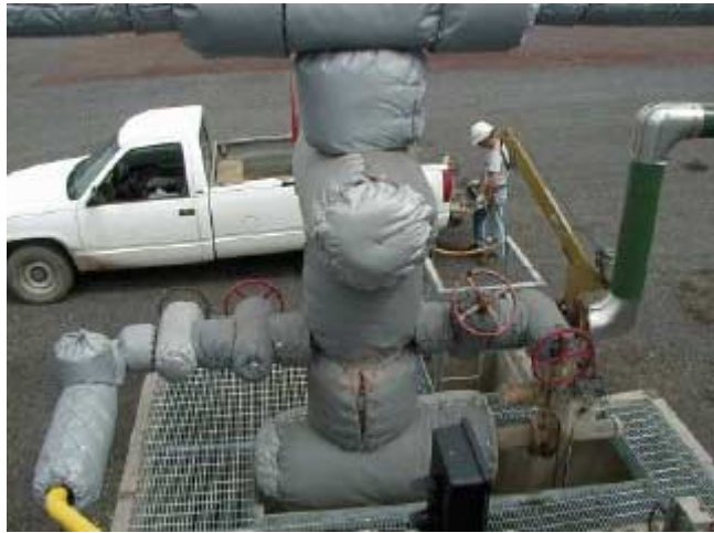
Figure 7 - Puna Wellhead Structure
