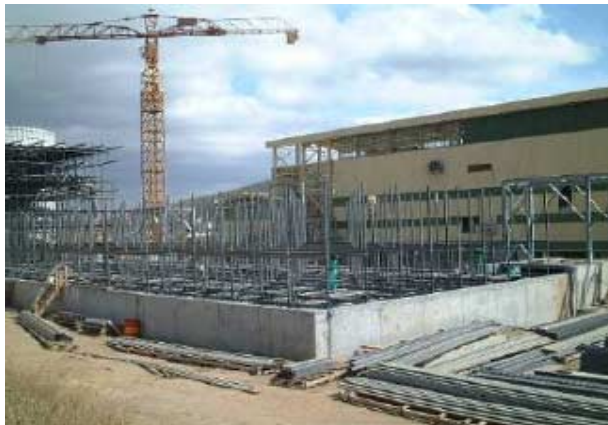
Figure 4 - Olkaria II Project
